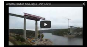
Tomorrow on cnplus.co.uk, read the full report and hear more about the challenges faced on the viaduct when Construction News went to see the Almonte Viaduct being built by FCC first-hand.
