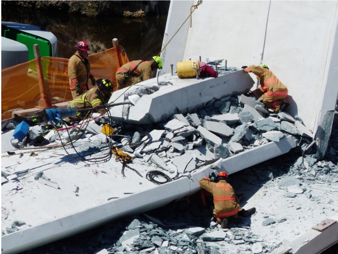
Collapsed end of florida bridge close up of blue jack pa
