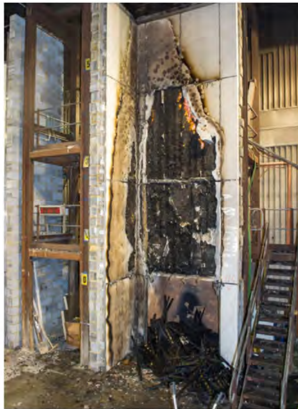
BS 8414 test on K15 with ACM, test terminated after 28 minutes (Picture: BRE)
