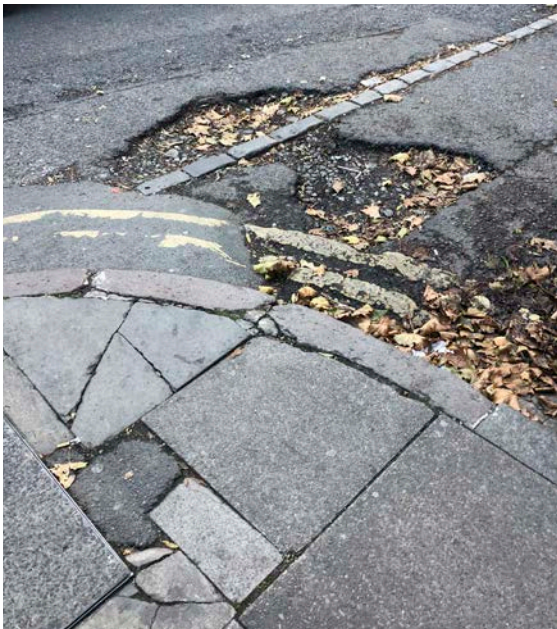
Paving on the Islington side of York Way suffers from disrepair. Photo: Nitasha Kapoor
