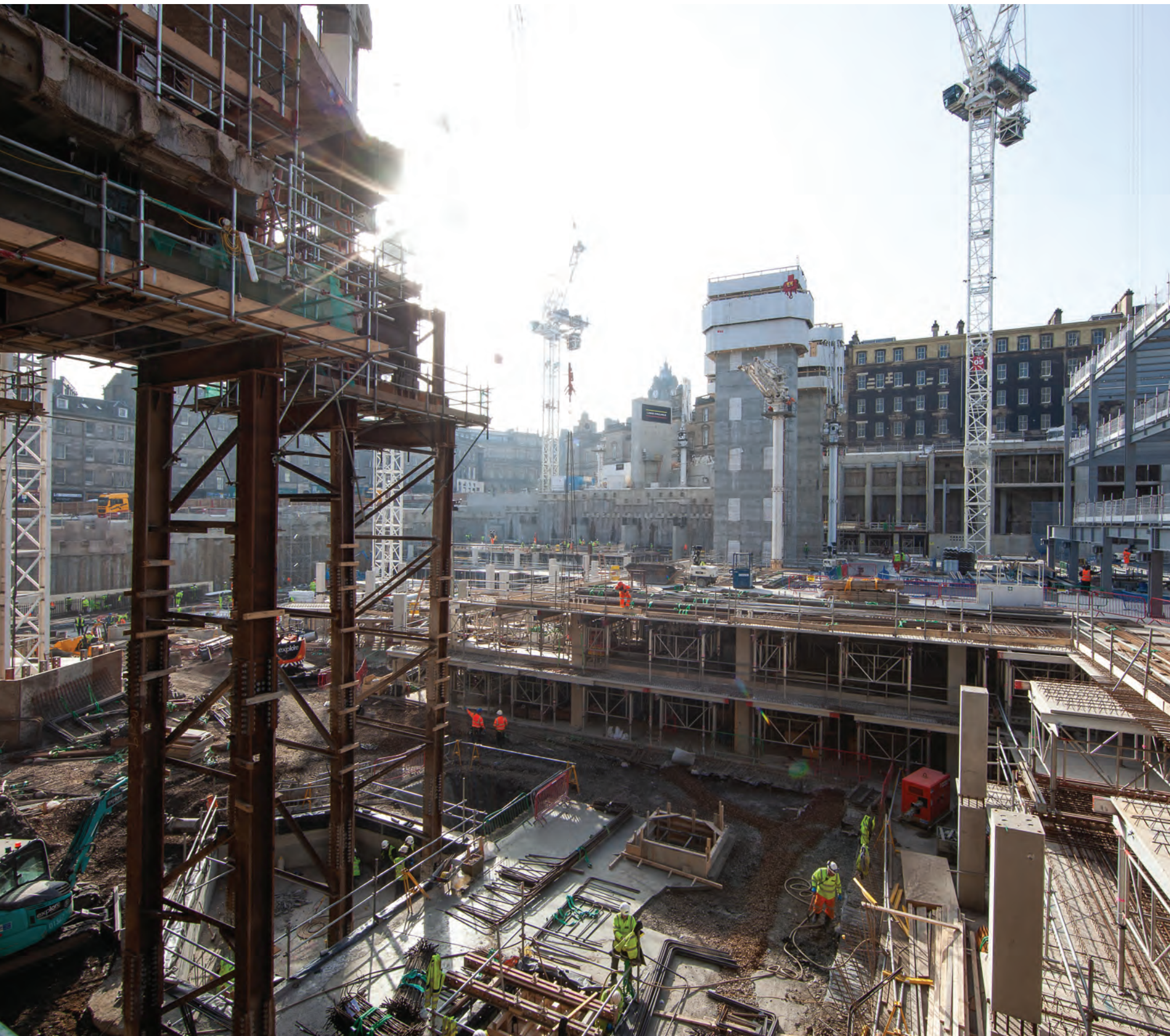
The Edinburgh St James site is in the city's New Town area and is hemmed in by buildings, roads and people. The job is complicated by having to work around and under a John Lewis store that extends into the site (on the left side of the image)
